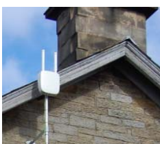
Discreet femtocell attached to a roof in Newcastleton
